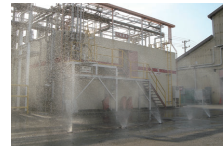
Yokkaichi Branch: Water Curtain System
