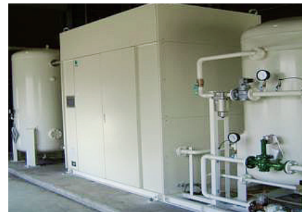
Shiga Branch Nitrogen Generator
