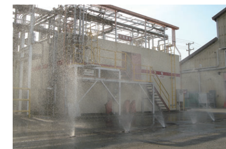
Yokkaichi Branch: Water Curtain System
